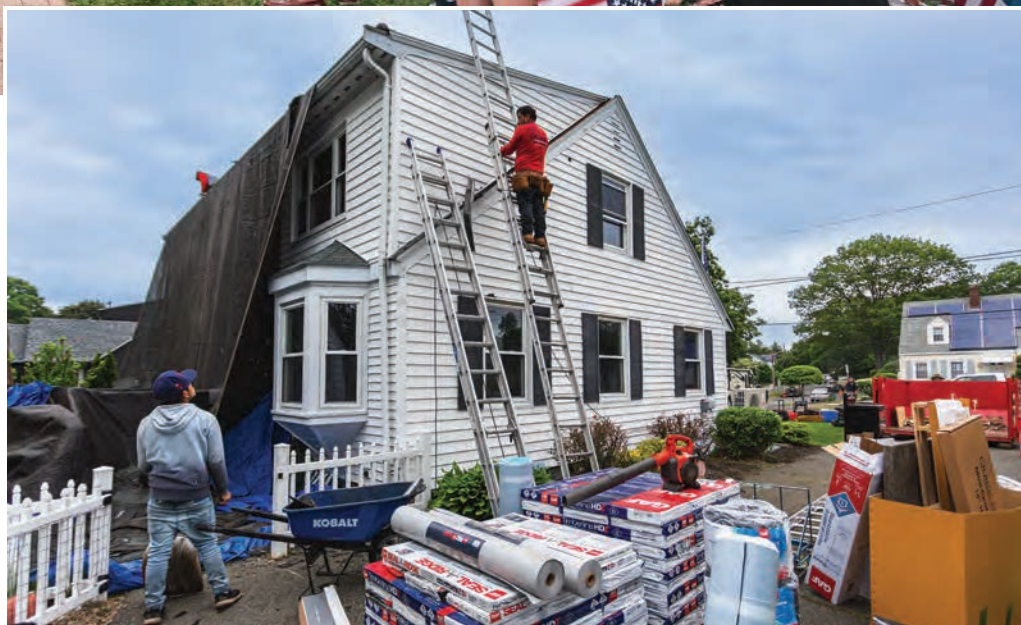
The Carmody family is welcomed back to their beautifully renovated home in Lynn, Massachusetts, during the 35th season of Military Makeover . (top, left) The Carmody family's home in Lynn, Massachusetts, undergoing a stunning transformation on the 35th season of Military Makeover . (above)
